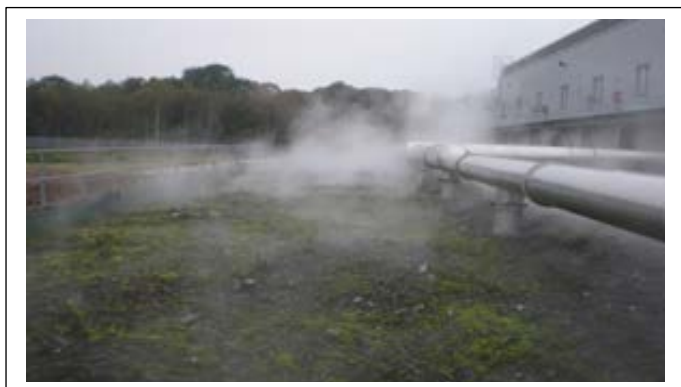
Open biofilter at a biowaste site showing the biofilter media surface and the arrangement of the inlet duct
